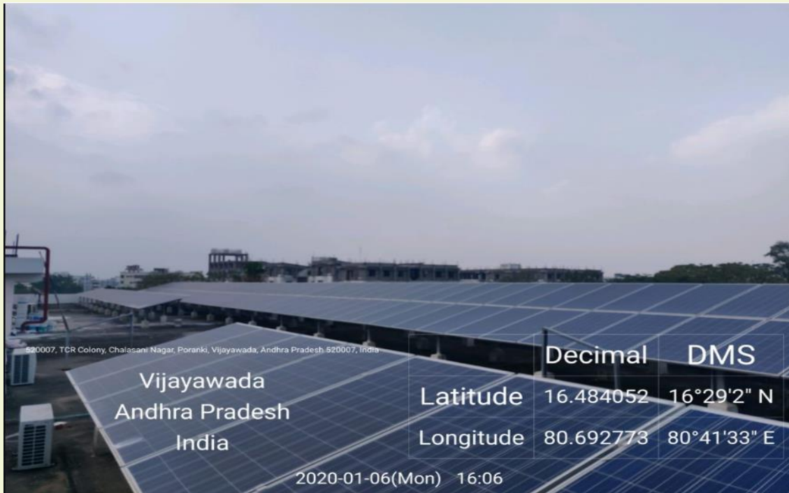
Solar Panels - Admin Office
