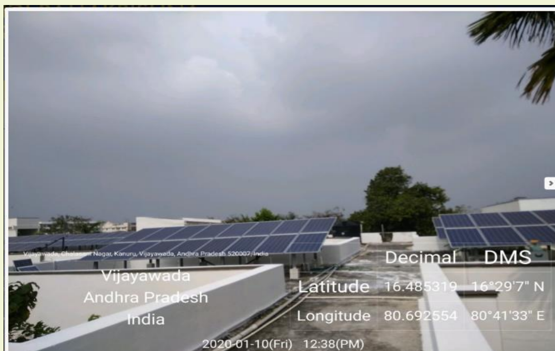
Solar Panels - EEE Dept
