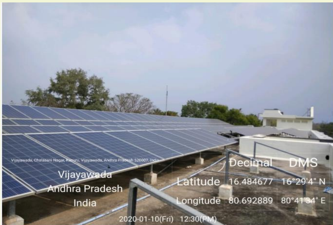
Solar Panels – S&H Dept
